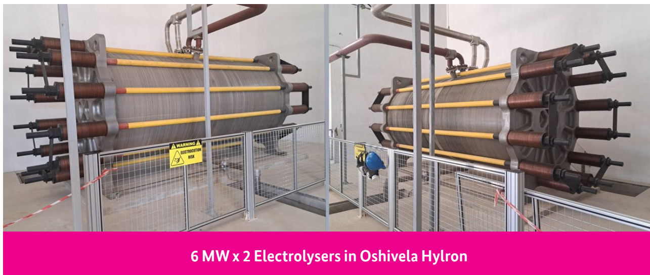
Figure 4: Electrolysers at Oshivela HyIron
