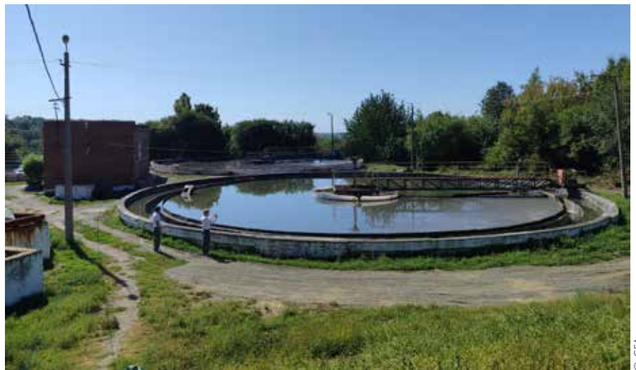
Industrial sewage treatment plant for water treatment
