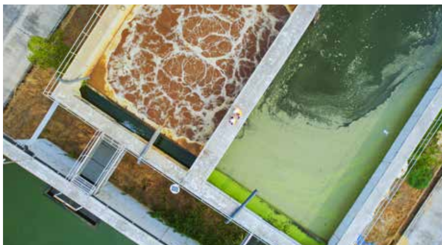
Industrial wastewater treatment plant
