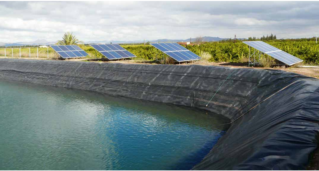
Solar Powered Irrigation System implemented in Morocco
