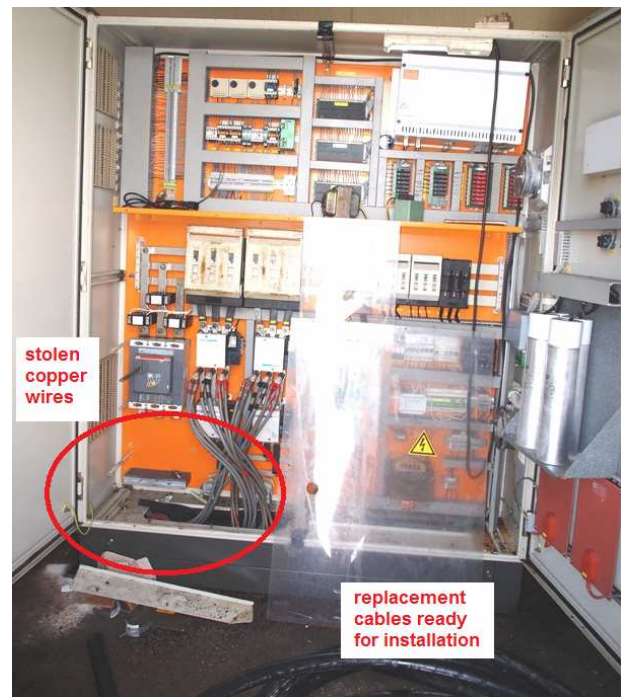
Figure 2-141: Stolen Copper Conductors
