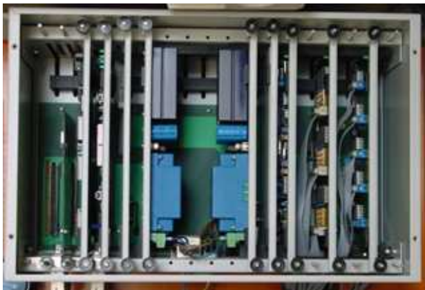
Figure 2-140: Burned-Out Controller of Nedwind 500 kW Inside of Turbine Controller before ...
