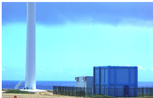
Figure 2-147: Vader Piet Aruba – Substation
