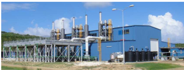
Photo: Vincent Kooij, “World’s largest hybrid wind-diesel power plant”, op. cit., slide 47
