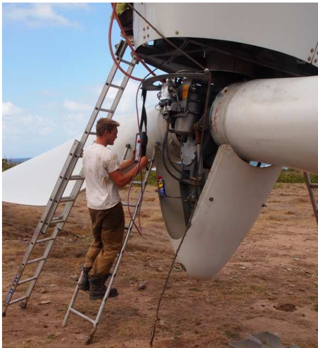
Figure 2-108: Using the “Copy Panel” of the Turbine Controller for Maintenance
