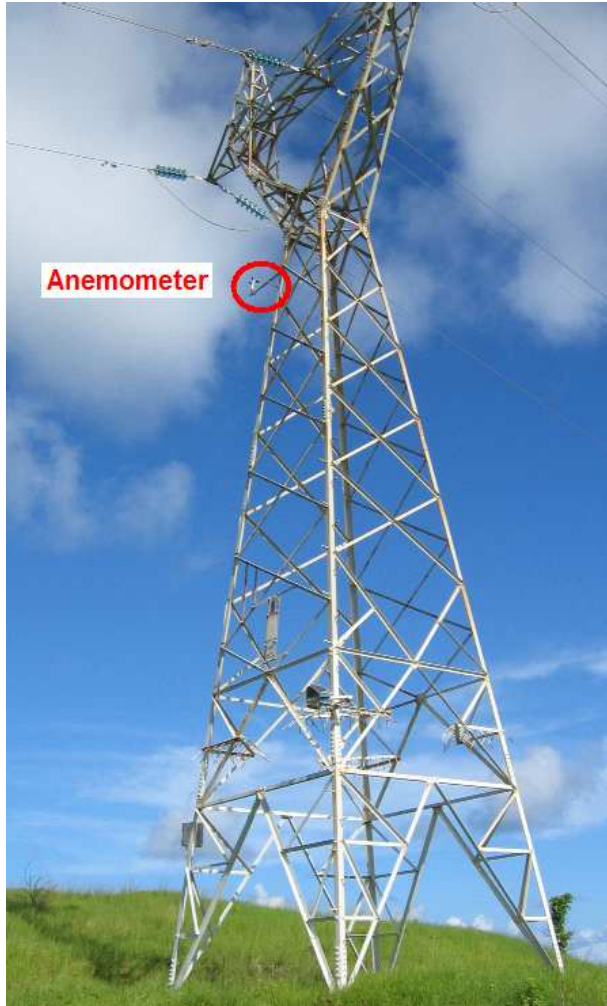
Figure 2-125: St- Lucia – Wind Measurements at 66 kV Mast
