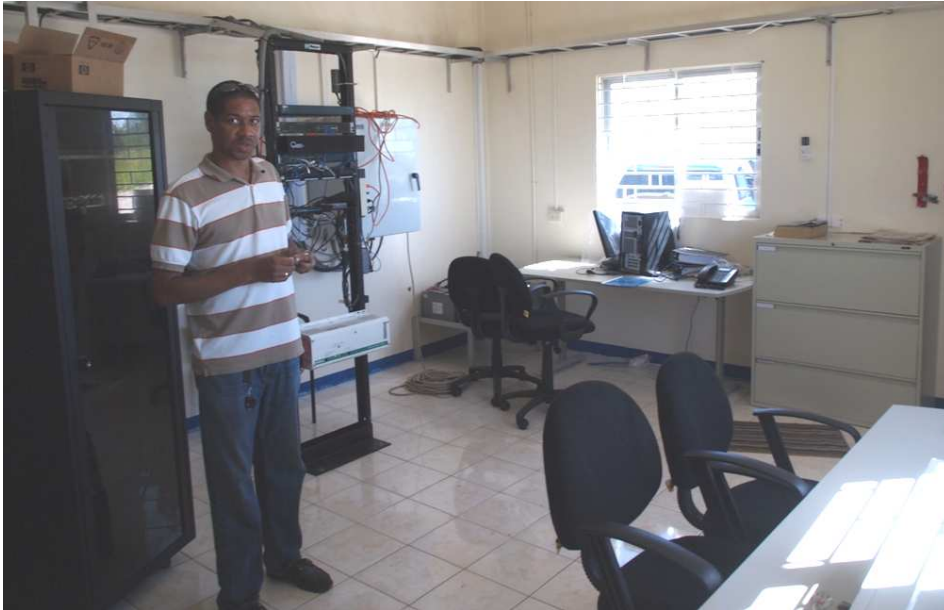
Figure 2-16: Munro Wind Park – Control Room in the Grid Station with Telecommunication and SCADA Equipment
