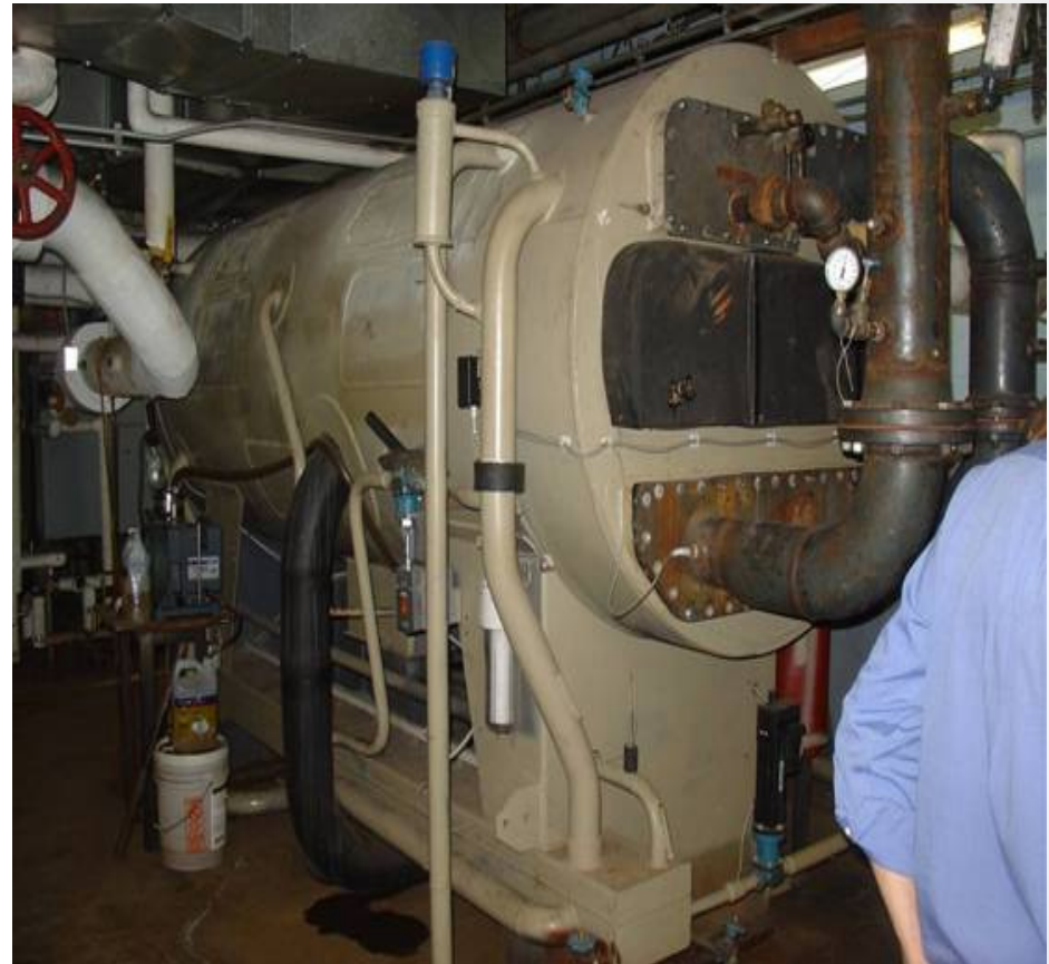
70 year old absorption chiller at University
