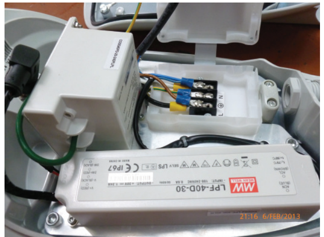
well-structured electrical components
