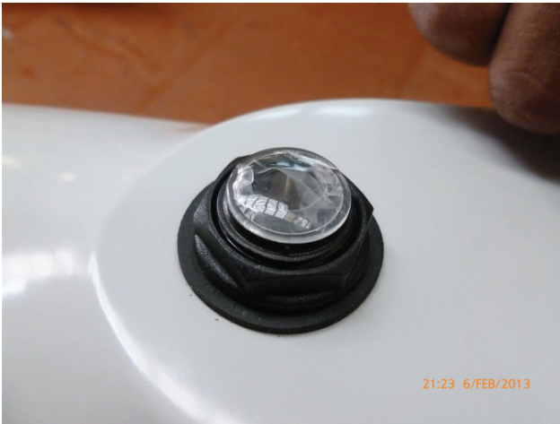
luminaire supplied with a broken photocell
