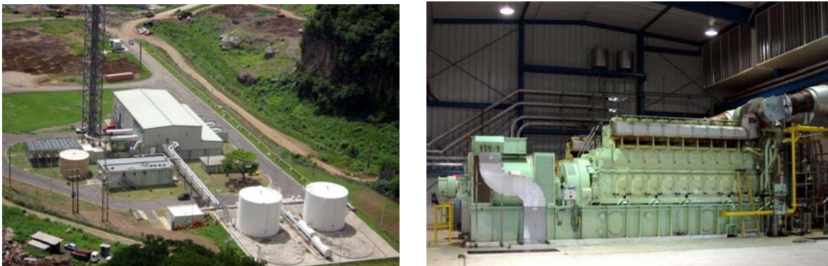
Figure 3.10.: Lowmans Bay power station with MAN 9L 32/40 engine [Source: MAN Diesel and Turbo]
