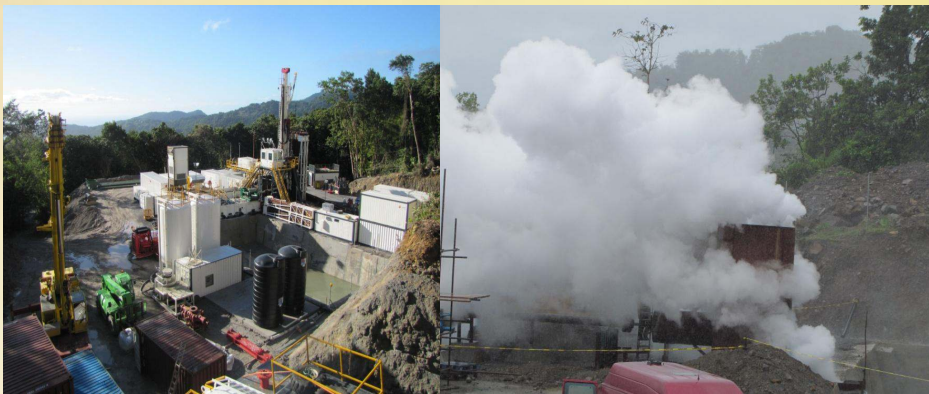
Geothermal development in the Roseau Valley area, Dominica
