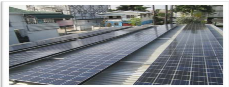
Solar panels mounted on the container shed in GEA's compound
