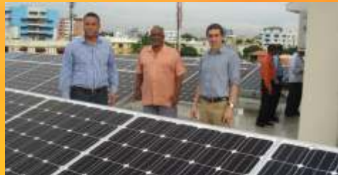
22 kWp PV Installation on CNE Building
