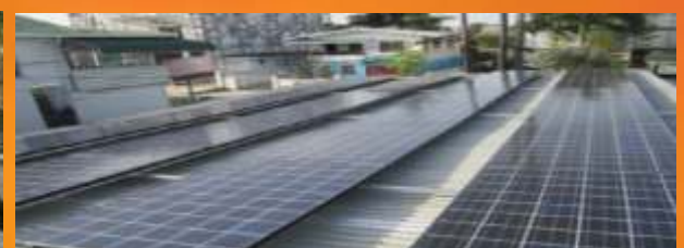
8.6 kWp Solar PV Installation at Guyana Energy Agency, Guyana
