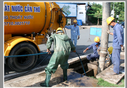
Regular cleaning of manholes can only be ensured provided sufficient revenue from wastewater tariffs.
