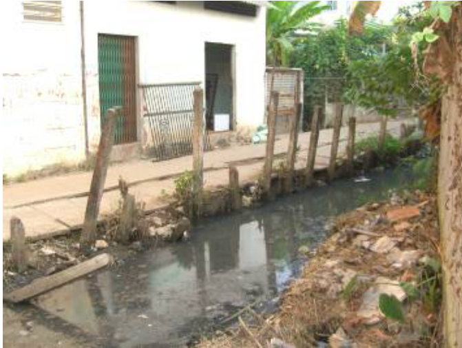
Photo 4: Natural ditch to which household wastewater is discharged – An Nghiep Ward
