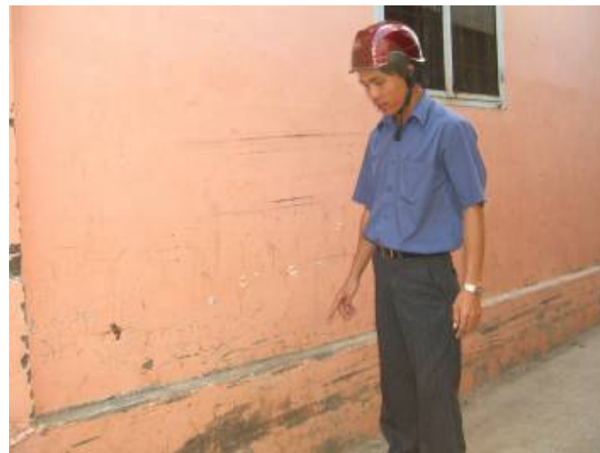
Photo 7: Ground level is low inside the area causing household wastewater can not discharge to main public drain but to natural pond – Ward 7
