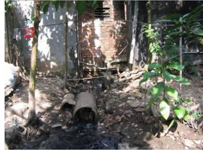
Photo 6: Natural ditch to which household wastewater is discharged – An Nghiep Ward
