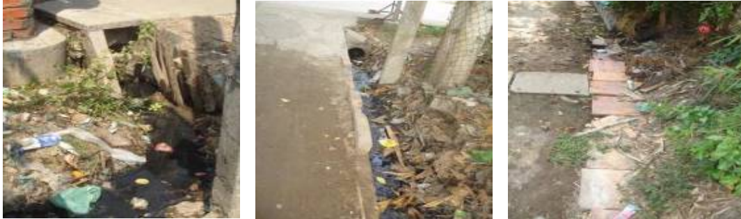
Small size of sullage pits/ drains in the alleys
