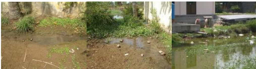
Waste water flows freely to the ground/ the nearby pond
